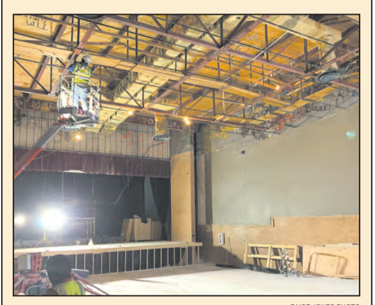
Names illicitly painted on the beams of the "catwalk" surrounding the MHS auditorium over the years have been exposed during the renovation project.
