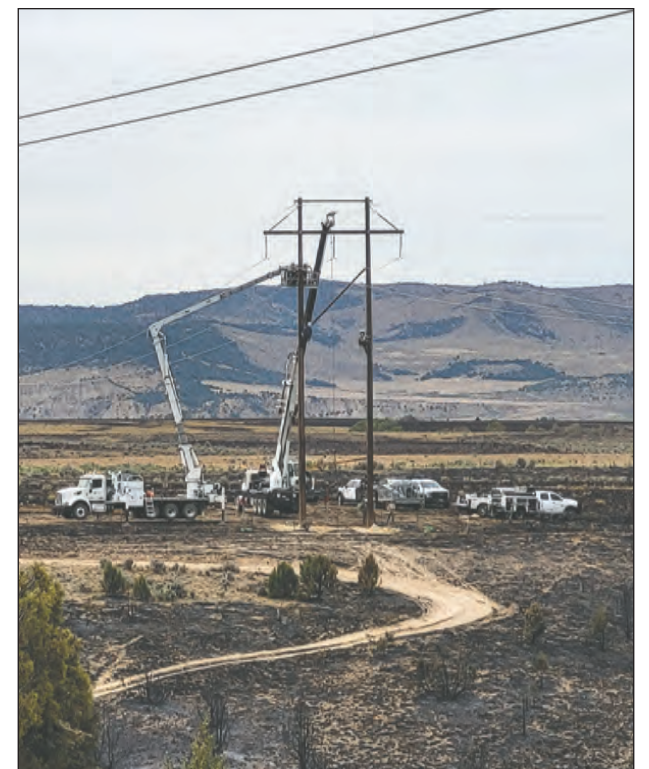
The post-fire recovery process entails multiple entities and organizations, including White River Electric Association, which was out repairing power lines on the Lee Fire in Josephine Basin on Aug. 9. KATHLEEN KELLEY PHOTO
